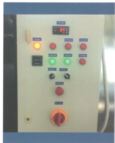
Electric panel for boiler device control
